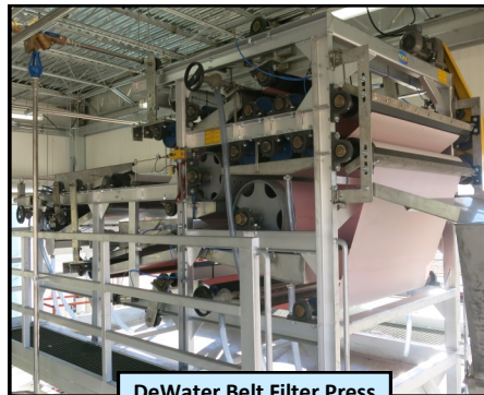
DeWater Belt Filter Press
