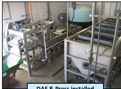
DAF & Press installed
