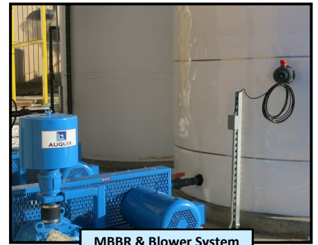
MBBR & Blower System
