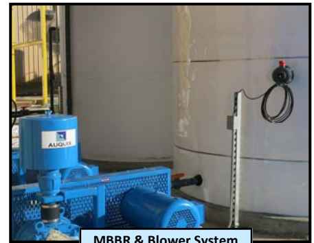
MBBR & Blower System
